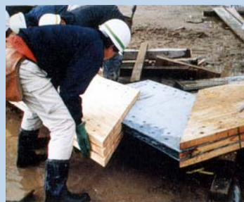
Dowelled or bolted joints with steel fin plates sandwiched between LVL or glulam members
