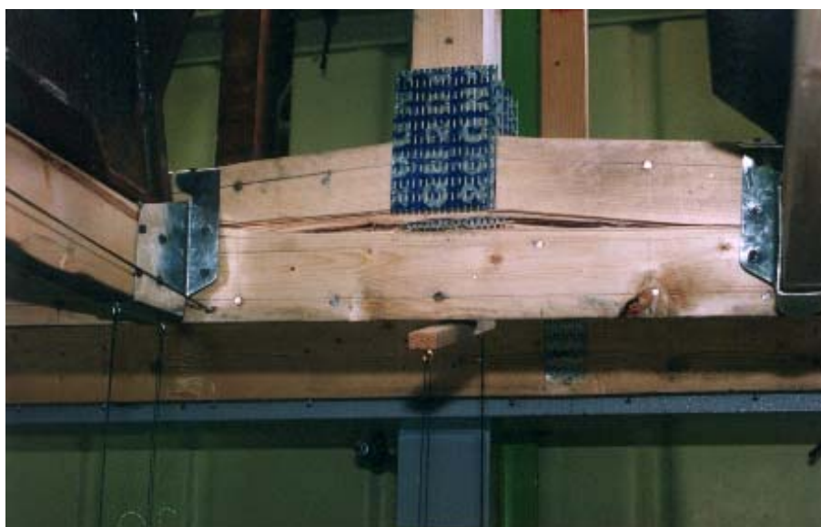
Figure 10: Typical tension perpendicular failure at the nodal points of girders
